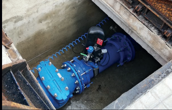
Example of an Installation in a Manhole
